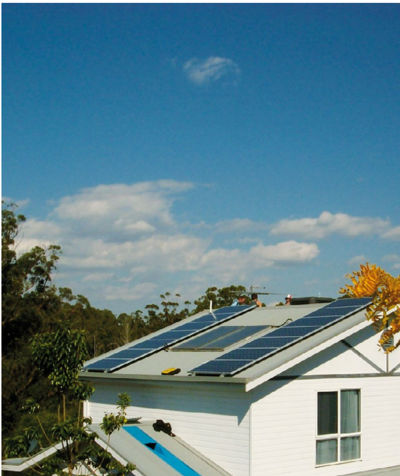
Reference installation in Gembrook (Victoria, Australia): 2.66 kW nominal output power - 14 modules - 1 SOLIVIA 2.5 AP G3 TR string inverter.
