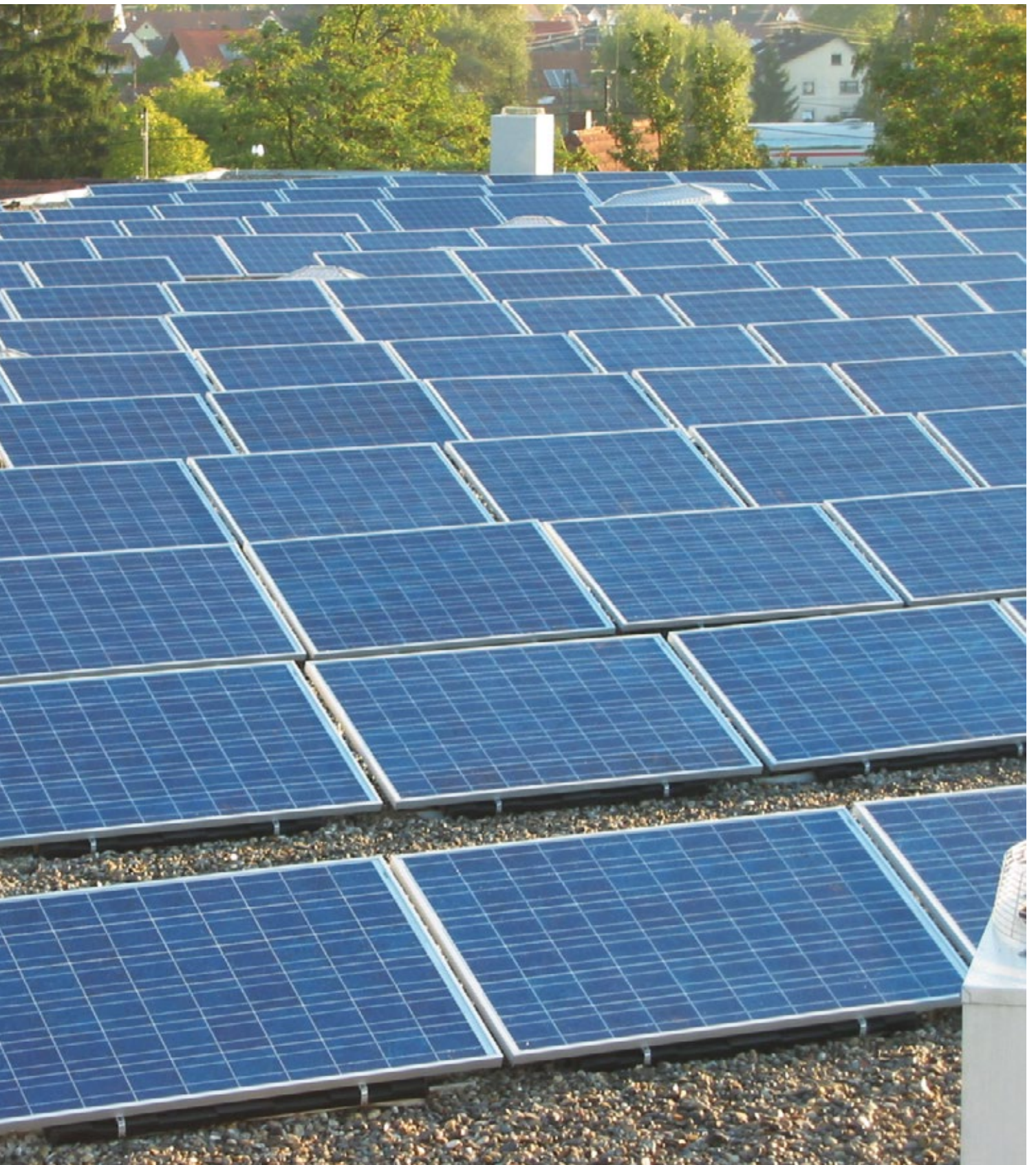
Photovoltaic installation at Delta in Teningen (Germany, Europe): 46 kW nominal output power – 205 solar modules – 15 string inverters.
