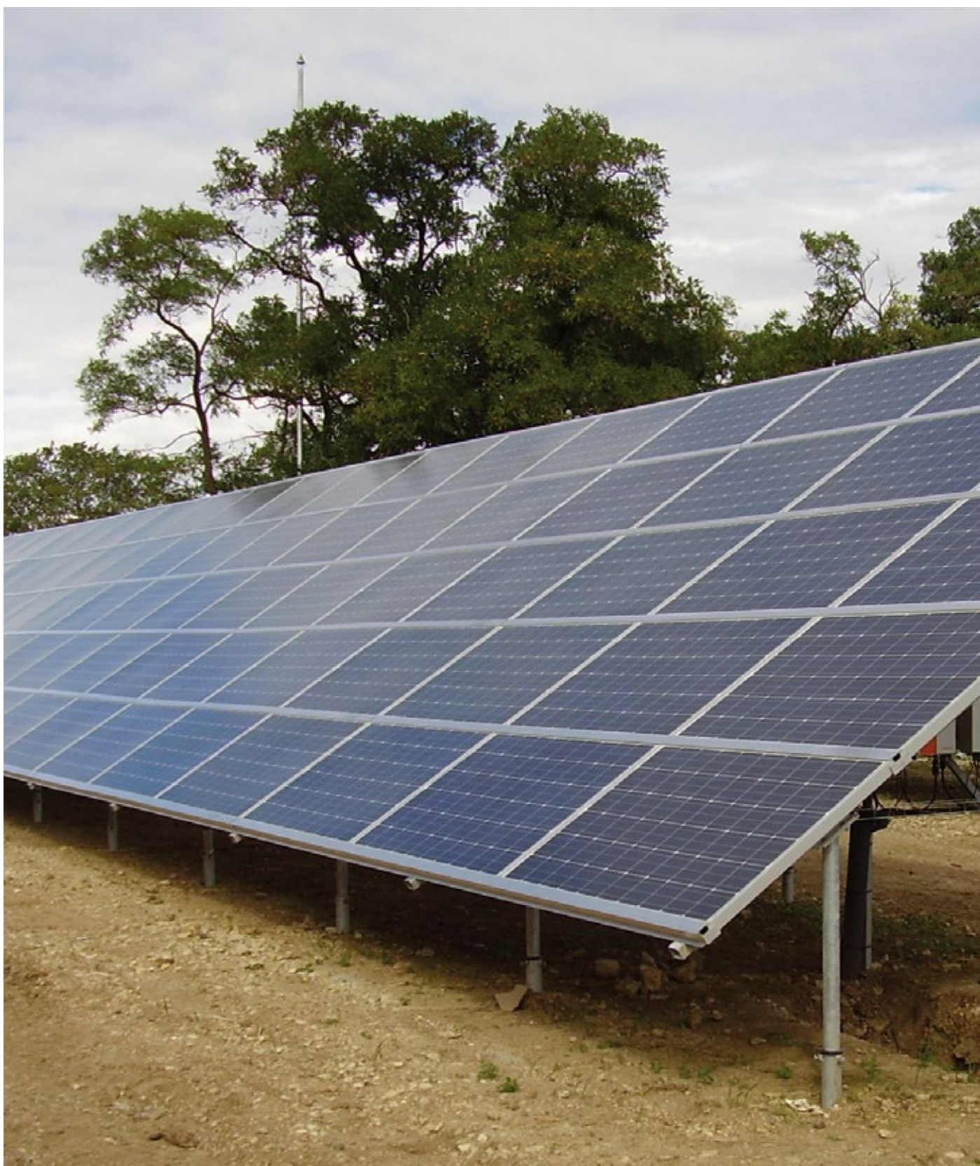
Reference installation in Vrapice (Czech Republic, Europe): 1 MW nominal output power - 4320 solar modules - 180 string inverters.
