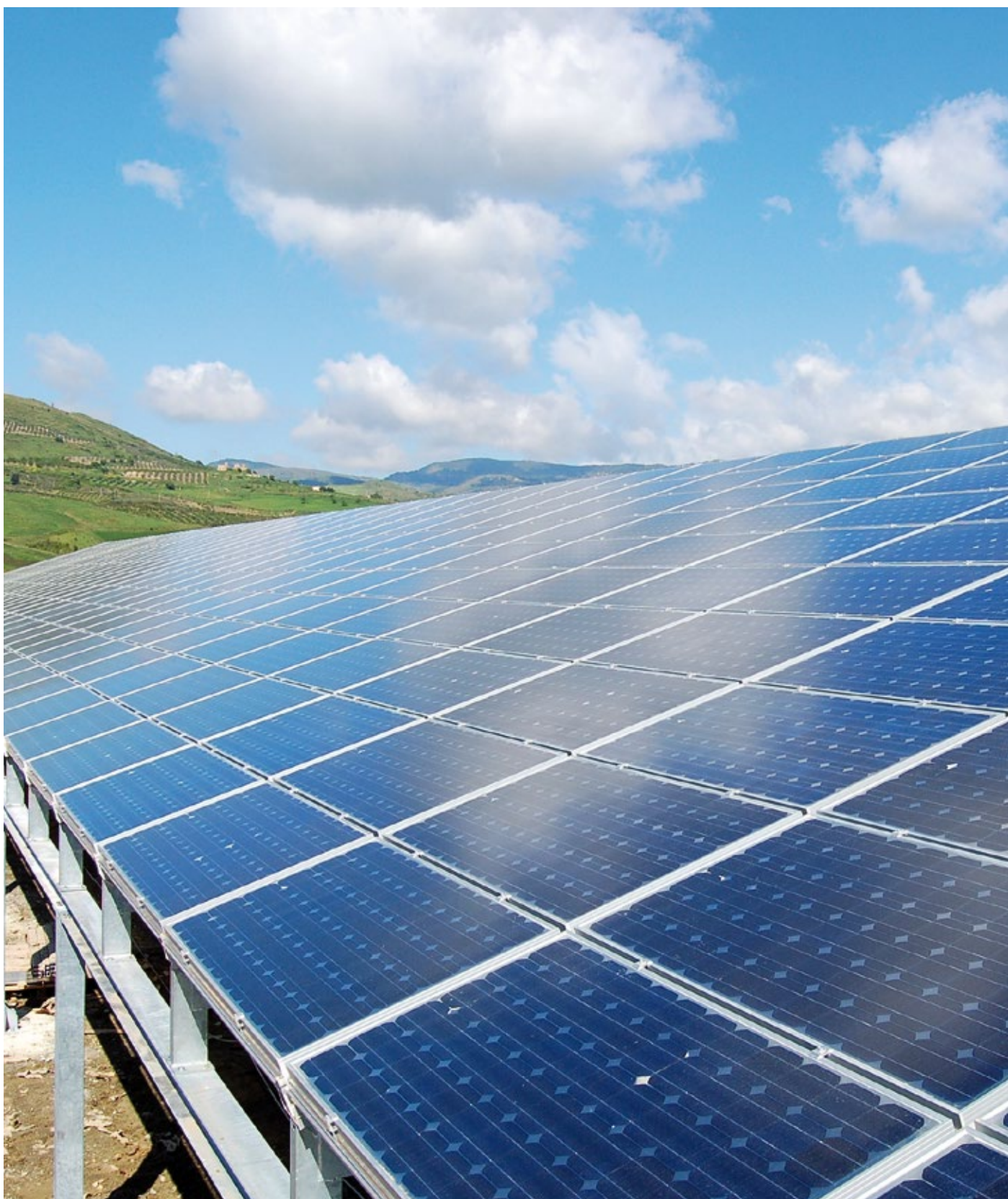
Reference installation in Bivona (Italy, Europe): 425 kW nominal output power - 81 string inverters.
